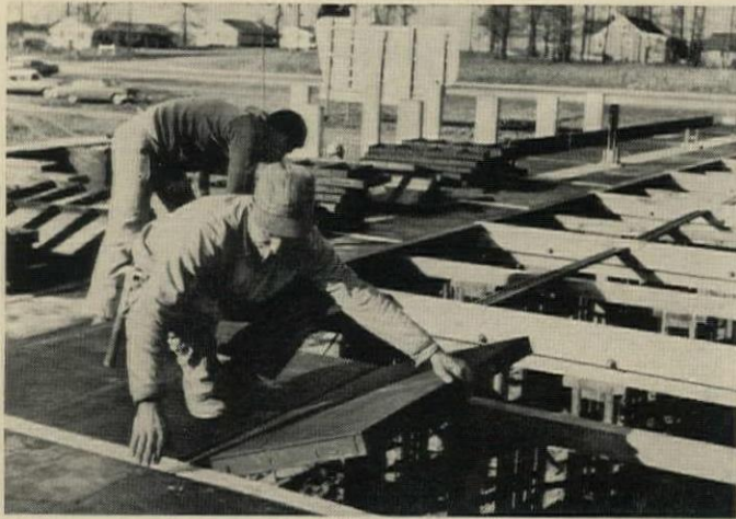
FORM IS SET UP by placing reusable panels so ends rest on shored-up wood beams. Panels are 4'x2' overlaid plywood on steel frames.
