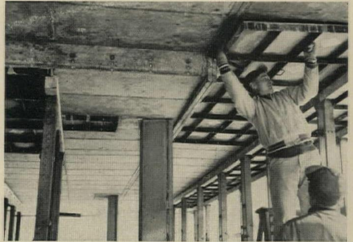
FORM IS STRIPPED by removing 4x4 support (see drawing) and sliding out panel. System permits work under a deck during pour.
