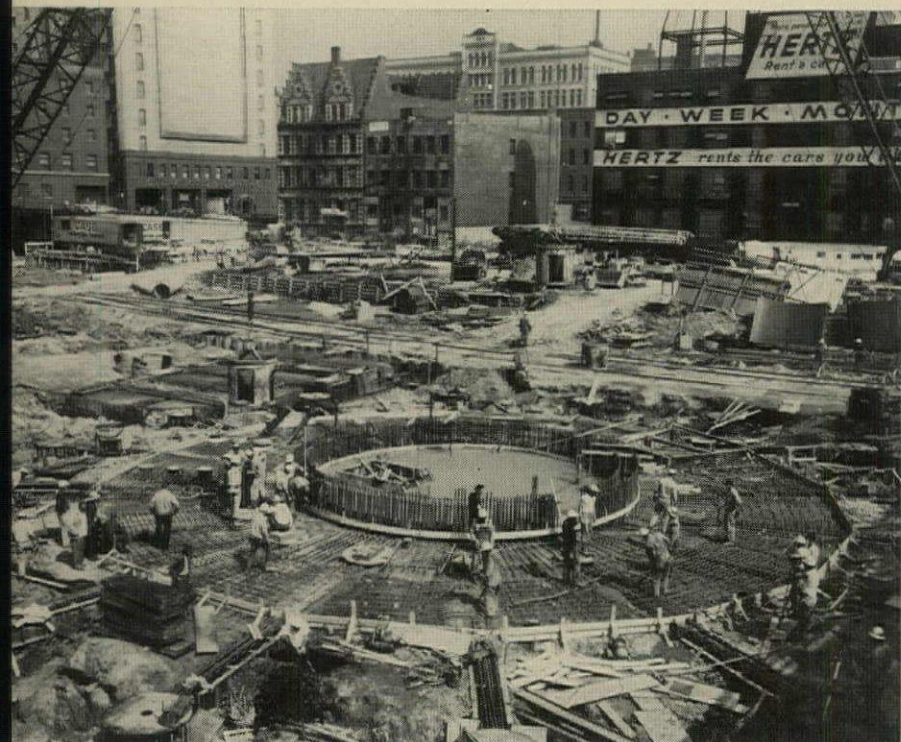
FOUNDATION reflects round design. Towers will be 105' in diameter, with a 35' central structural core housing elevators and utilities.
