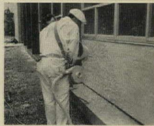
Modern machine application is efficient in applying finish coat and marble dash stucco and sharply reduces labor costs
