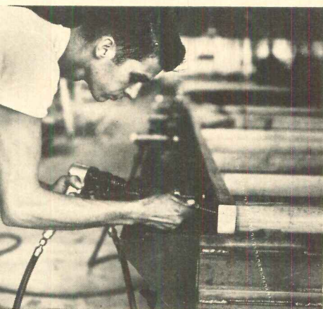
DRIVING GUN saves much labor time. Here it is used to nail sill of interior wall panel.
