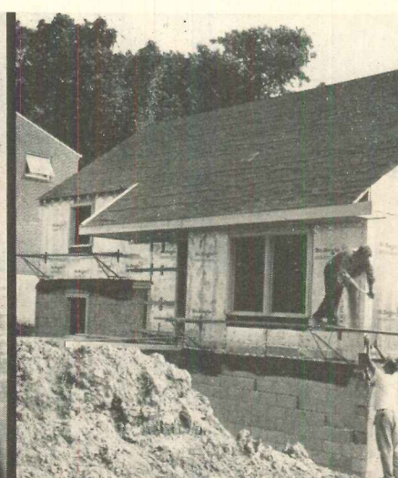
The completed house — literally wrapped in continuous insulating material — is glowing evidence on your building site of the extra value you are giving at a low cost.
