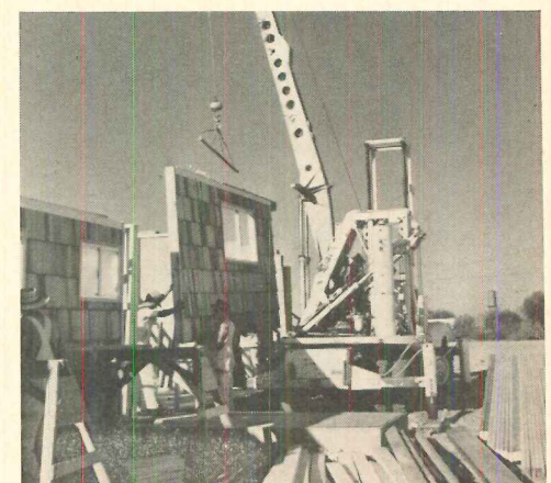
WALL TAKES SHAPE at rear of house as sections are added. Three panels extend 60' across house.
