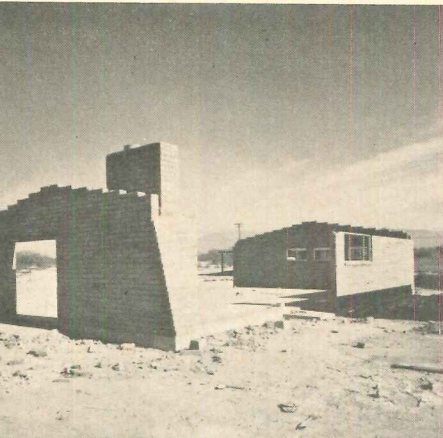
MASONRY WALLS are built with Mexican adobe block by subcontractor before components arrive.
