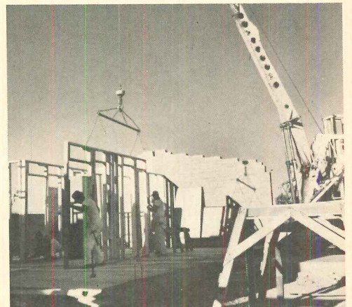
INTERIOR PANELS are unloaded one or two at a time, set on color-chalked lines marked on slab.
