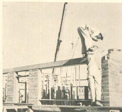
HEADER over window and door at front of house is set by two men who also erect carport beams.
