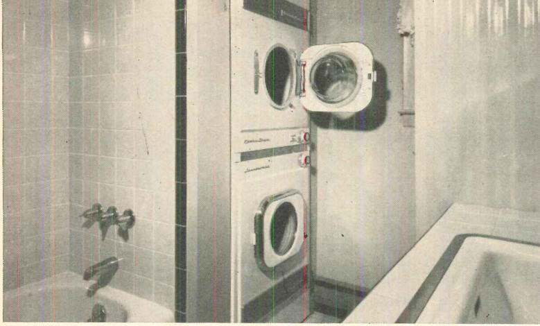
HOUSEWIVES appreciated having the washer and dryer in the bathroom. Stacked as shown, the Westinghouse Space-Mates fit in a space only 25 inches wide. A removable panel in a closet provided access for servicing.
