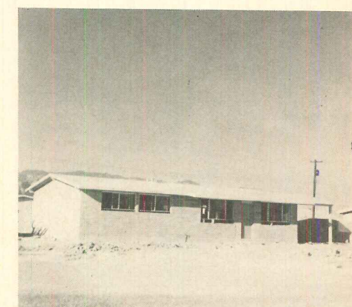
HOUSE IS CLOSED IN by eight men (including crane operator) 5 1/2 hours after components arrive.
