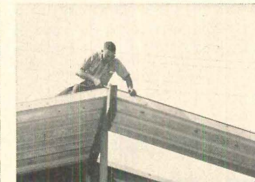
14 Roof panels are toe-nailed into ridge beam and wall plates. This is roof section over porch.
