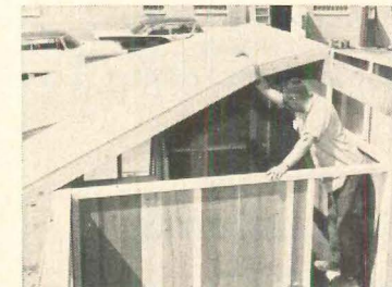
13 Roof panels (2x4 framing with insulating fiberboard deck) are set on side walls and ridge beam.
