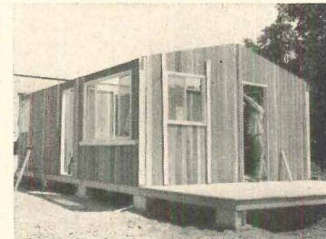
9 Job is at halfway point here. End floor panels, foreground, form porch. Siding has V joints.
