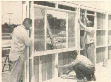
7 Front wall is erected. Windows are aluminum. Framing lets owner insulate and finish with drywall.
