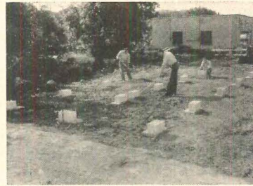
1 Concrete blocks are placed on precast pads dropped on ground for Harnischfeger house.
