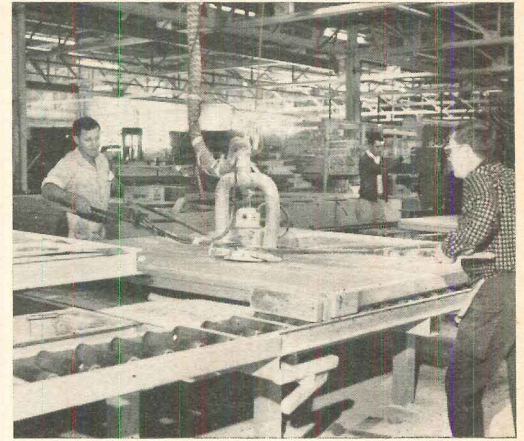
6 After drywall is nailed window and door openings are cut out by two-man router. Shoulder of router bit is held against the lumber frame opening and acts as a guide for correct size of the opening.
