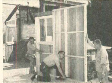
4 Wall panels (2x4 framing with vertical sheathing-siding) are nailed through plate edge of floor.
