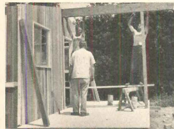
11 Double 2x12 ridge beam goes up, rests on porch column, end walls, and column in previous picture.
