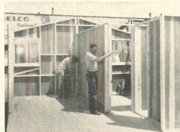
8 Partitions are installed. Doorsill framing, needed for handling, is cut out after erection.
