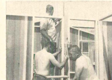
10 Column is installed between bedroom doors to support ridge beam. Bathroom door is at right.
