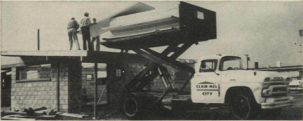
HOUSEFUL OF ROOF PANELS is lifted at one time by a Tampa builder's flatbed scissor truck.
