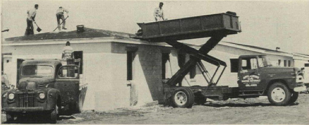
BUILDING PAPER, TAR AND GRAVEL are raised to roof by Orlando subcontractor's scissor-lift.
