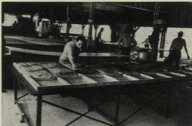
PANELS ARE SHOP-BUILT. First, 2x2 purlins are laid out on jig table, 3/8" plywood outer skin is nail-glued. Then panel is flopped over, insulated, and 3/8" drywall interior face is glued in place. Uninsulated section of this panel will form roof overhang, have Upson-board face.
