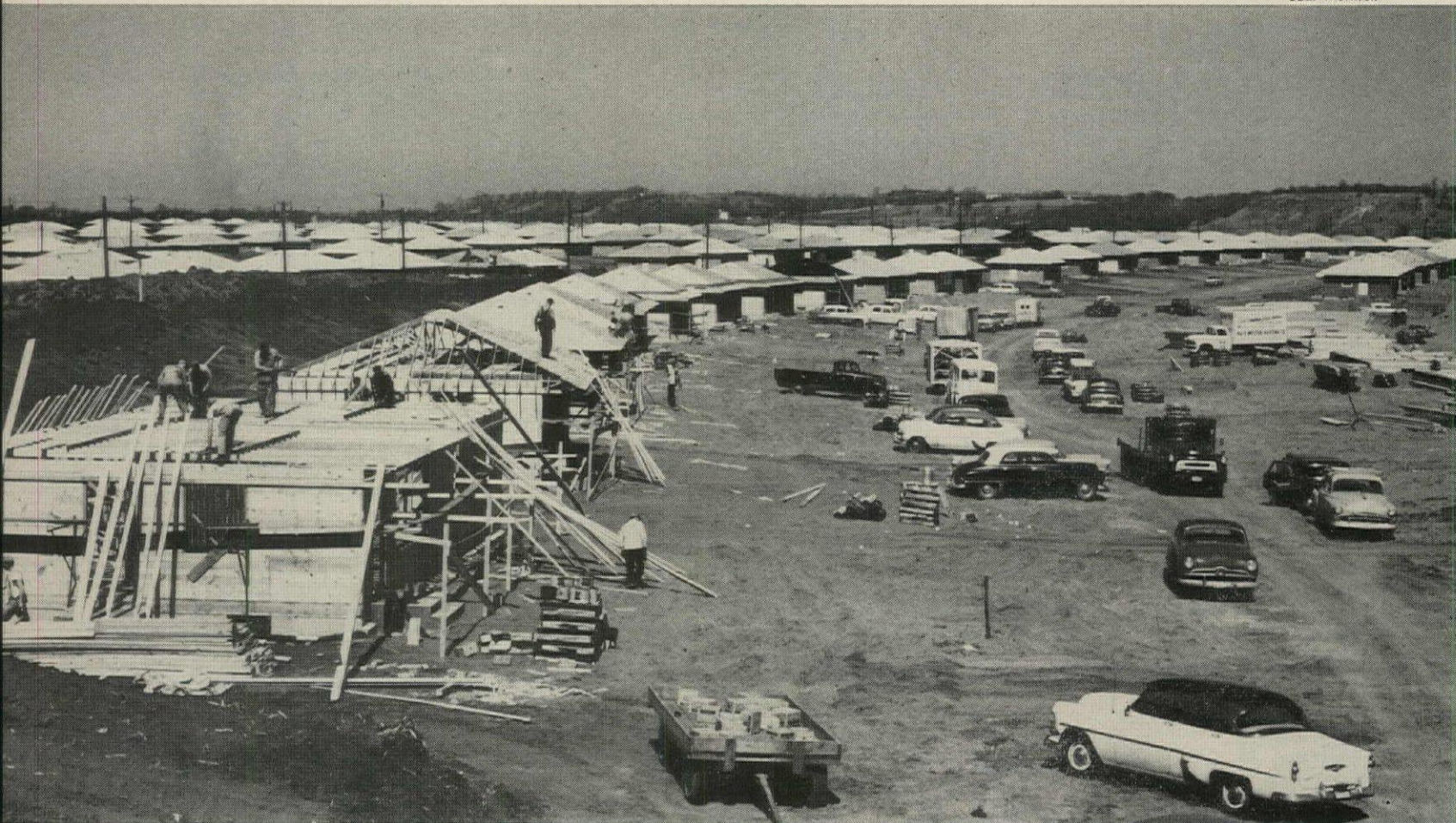
HOUSES ARE BUILT CONVENTIONALLY, but under Thompson's system not a man-hour or a 2x4 is wasted. Note material stacked for use.
