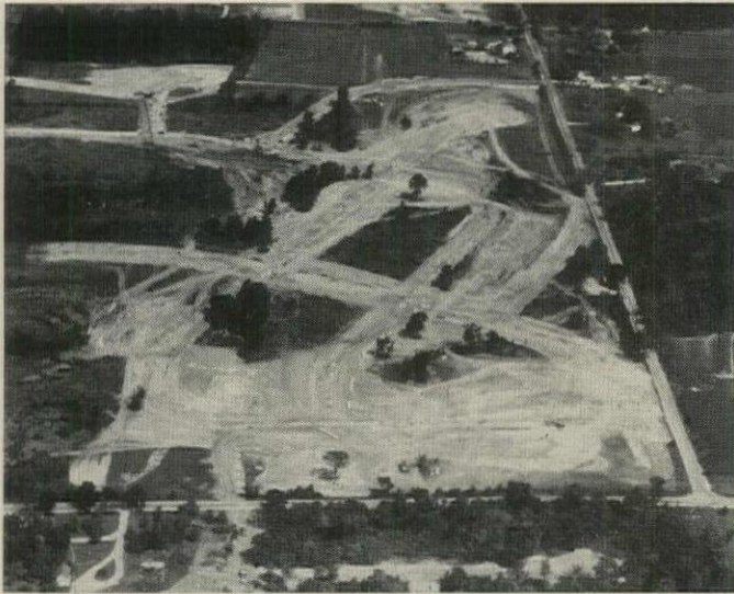
BEFORE houses go up, La Bonte grades sites; puts in sewers, curbs, gutters. This is part of his Edgerton Highlands subdivision in Greendale.
