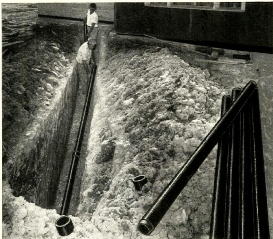
A Permaline fibre pipe house-to-street sewer installation by N. J. Rodrigue, in a home project at Houma, Louisiana. Builders all over the country have found Permaline economical, profitable to install.
