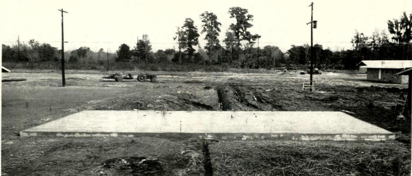
FINISHED SLAB awaits framing crew. Slab construction is not in 14-day building schedule.
