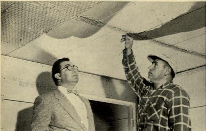
Eby (left) inspects application of Keycorner, used to reinforce joints. Keycorner is also used at all wall and corner junctures.
