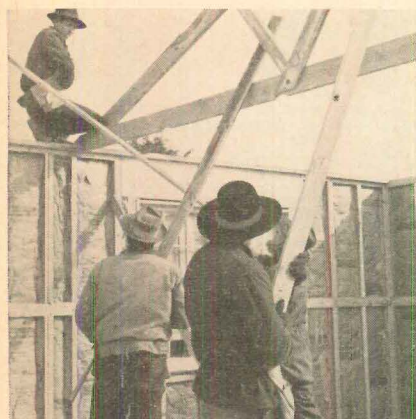
SELF-SUPPORTING TRUSSES —American Houses' fink-type split-ring trusses require no support. Inside partitions carry no load. Walls and partitions are notched for quick, accurate spacing.
