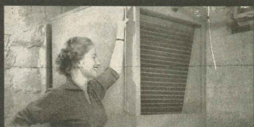
Here H&M Residential Unit is installed in small chamber under front steps of home.
