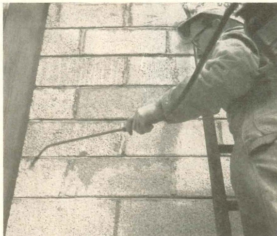
Silicones do not change the appearance of masonry. Photograph shows how a silicone water repellent is applied to a block wall with a low-pressure spray. Within two to 12 hours the solvent evaporated, leaving a smooth, protective film over the exterior surface.
