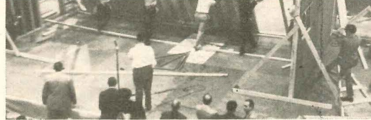
Up she goes! Crew tilts wall into place between waiting side walls.
