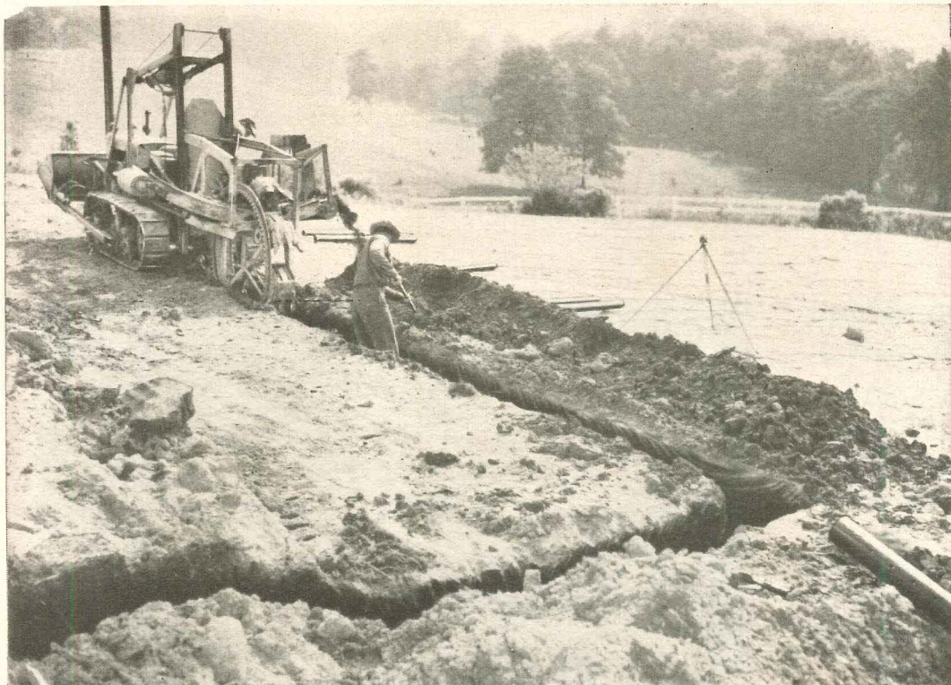
A land-drainage installation of perforated Perma-Line pipe on the J. L. Shannon estate near Detroit. Photo Courtesy Superior Tank Company.
