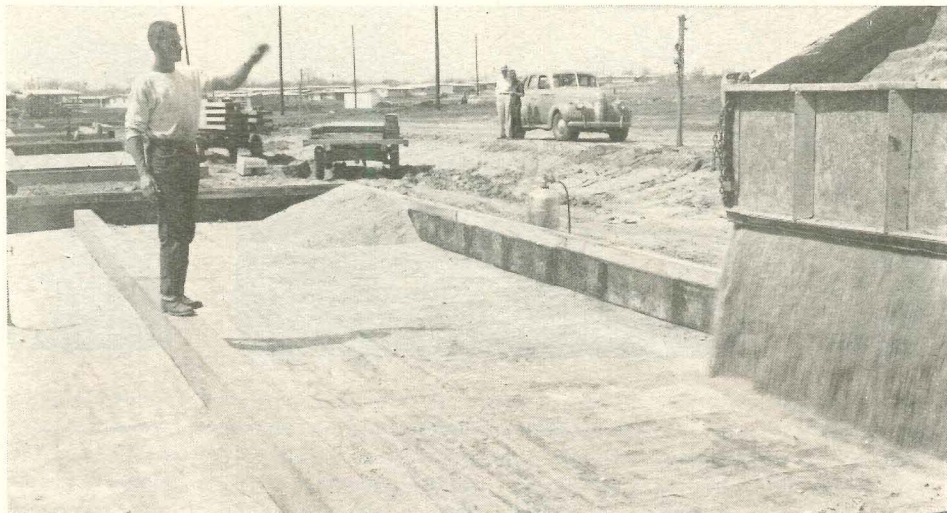
Membrane moisture barrier is well lapped, then covered with 2" of washed gravel to hold it in place. Four-man crew can prepare five foundations per day (spread footings is a separate operation). Chief reason that Strauss is able to move stem wall forms so quickly is stiff slump concrete; 4-to-1 curb mix is well rodded into steel form, takes on initial set in 2 hours.
