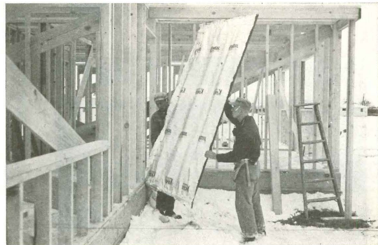
The sheathing is then nailed to the stud exteriors as usual, the insulation compressing to 3/64" under the studs. U factor of this wall: .12.
