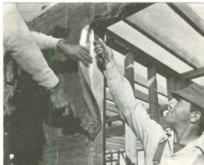
Blanket turns into window openings, acts as calking. Scraps become calking too.
