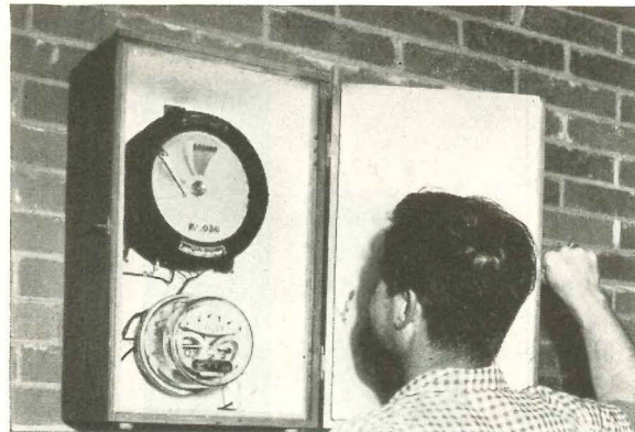
Special meters kept continuous record of electricity used for cooling each house. Other instruments recorded inside temperatures, humidities, air velocities, noise levels, etc. (The initial operating cost data released in Chicago contained errors for seven houses which were discovered later; H&H's $109 average, plus individual house bills given on pp. 156-157 are the corrected figures with allowance for the mistakes.)
