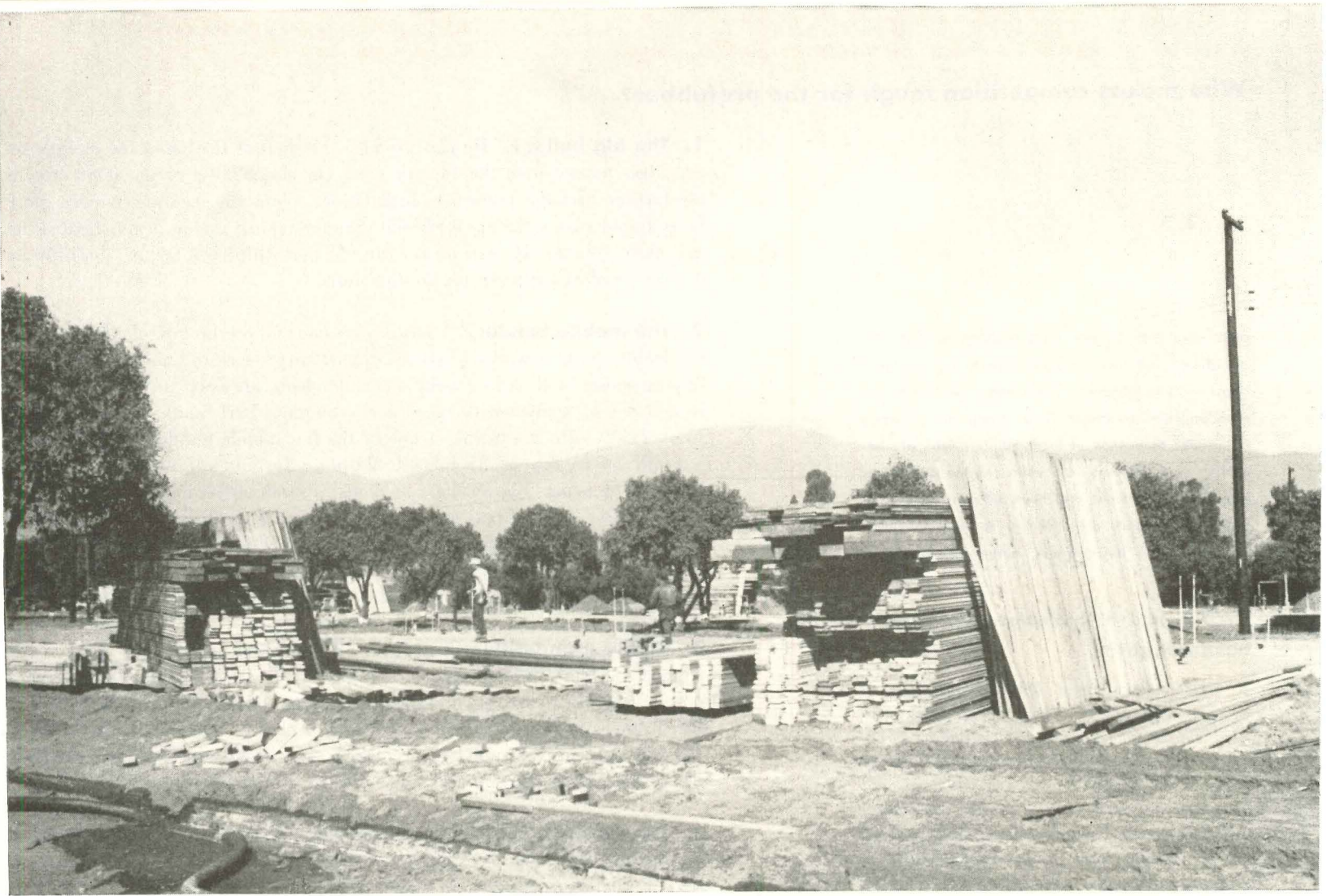
Precut lumber is unloaded near slab with pieces to be used first on top
