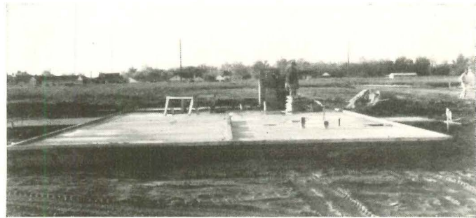
At 7 a.m. workman readied slab for prefabricated parts. Truck arrived shortly after; first framing panel was up at 7:15.
