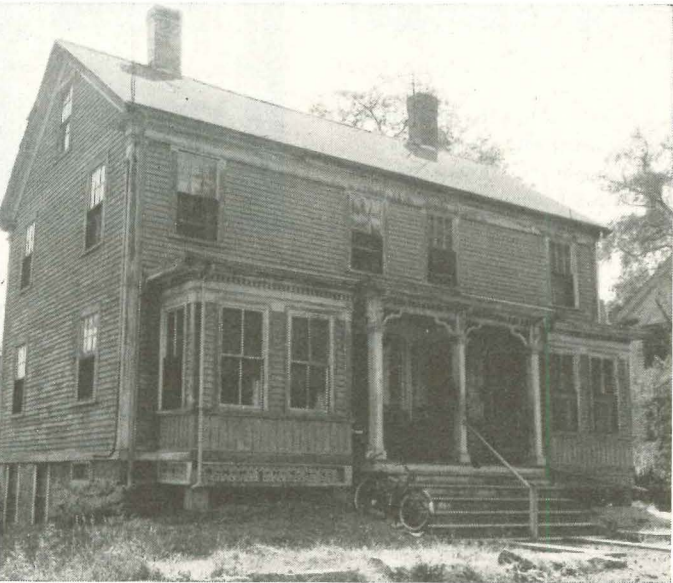
Before. Fast-decaying two-family house came to Turchon in an estate. In need of paint, dirty, rundown, it needed thorough overhauling. No one ever wants appraisers to see a house in this condition.
