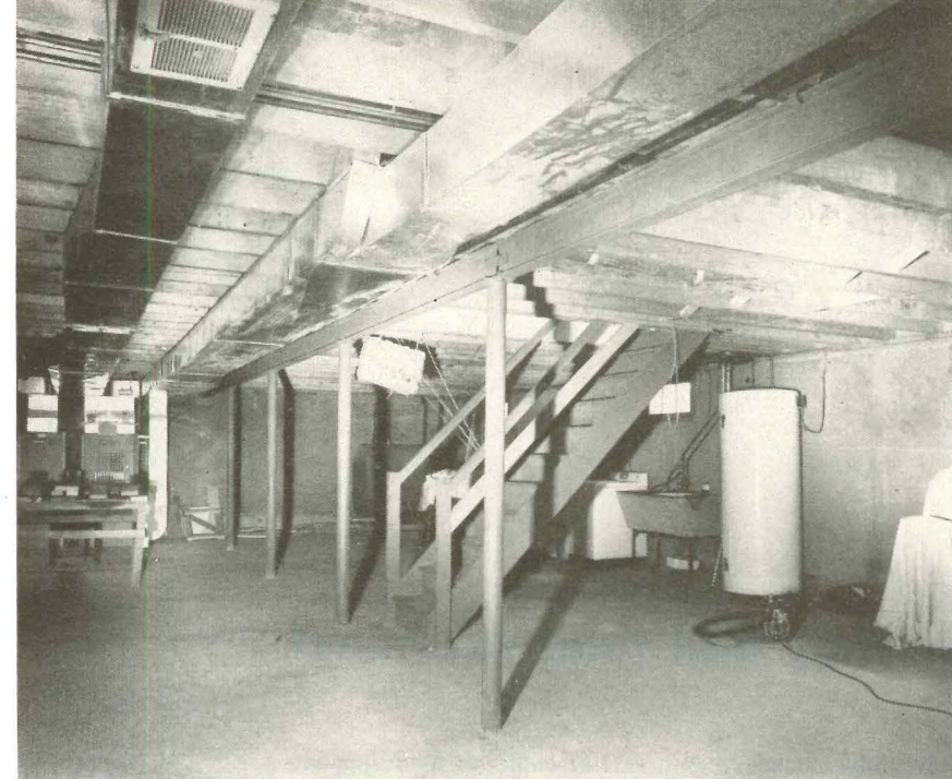
Before. Basement was unsightly with heating and cooling equipment, overhead ductwork, laundry appliances and tubs, hot water heater, various pipes and wires. Badly lighted space was used only as storage room and workshop.
