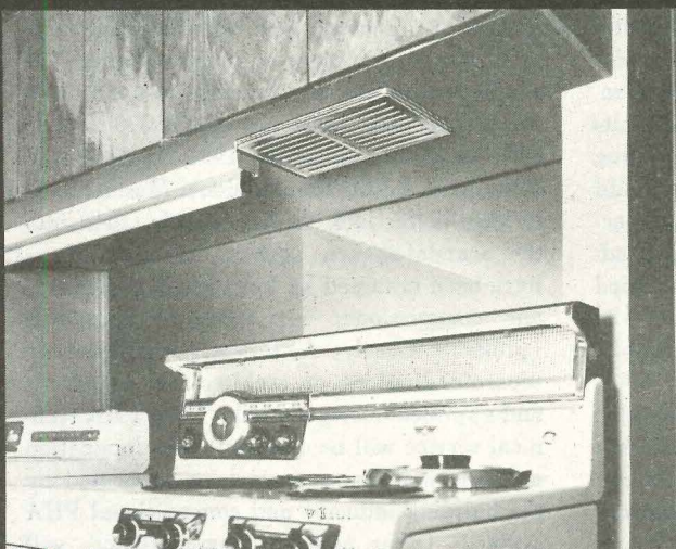
Builder W. A. Burns (Home #15) chooses a NuTone 870 Twin Blower for kitchen . . . and also a NuTone Ventilating Fan for Bathroom.
