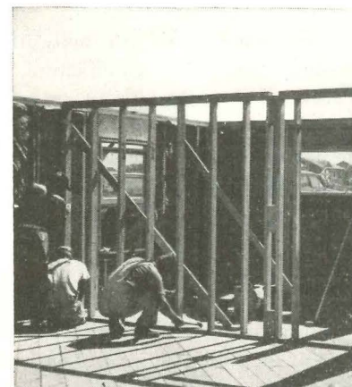
9:10 A.M. Carpenter crew sets non-bearing partitions before trusses are erected because workmen like it that way and found his "back of truck" system fit.
