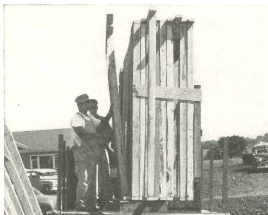
9:00 A.M. Preassembled interior partitions are moved into house through gap left in front wall where integral door and window wall will be placed after all the interior partitions have been erected.
