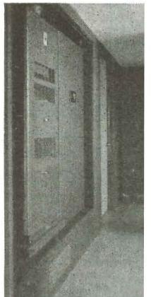
SUNBEAM HEATING units are located in utility room.
