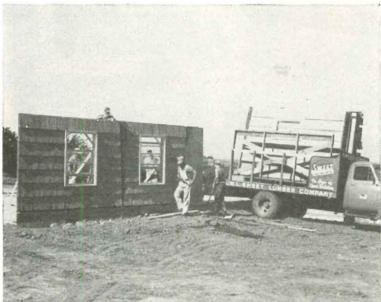
8:10 A.M. Labor force of five carpenters and two laborers has already worked ten minutes, put up two front wall panels. Ground was leveled so truck could back up to platform.
