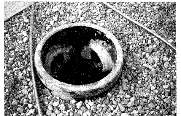
2. Sewer crock plenum and 6" tile ducts give fire- and rust-proof perimeter heating. Down-flow furnace discharges warm air directly into low-cost 18" dia. crock which can be bought anywhere. Unlike sheet metal, tile ducts do not float during pouring of slab, do not need concrete under them.
