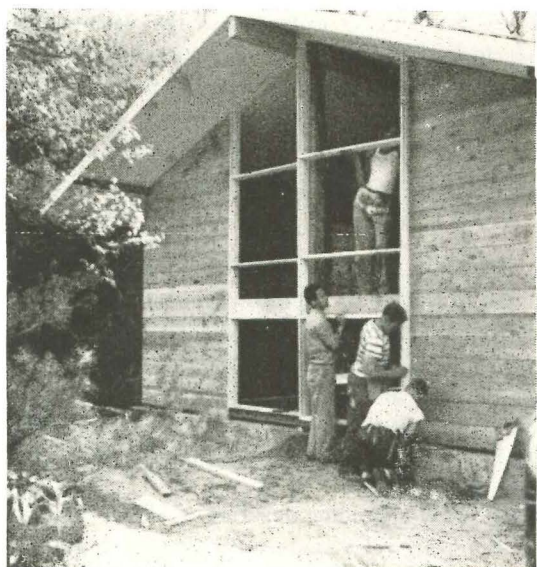
8. Uphill end of house, through which building materials have been unloaded, is closed in last. It has taken a six-man crew only 1½ days to get the house under roof.
