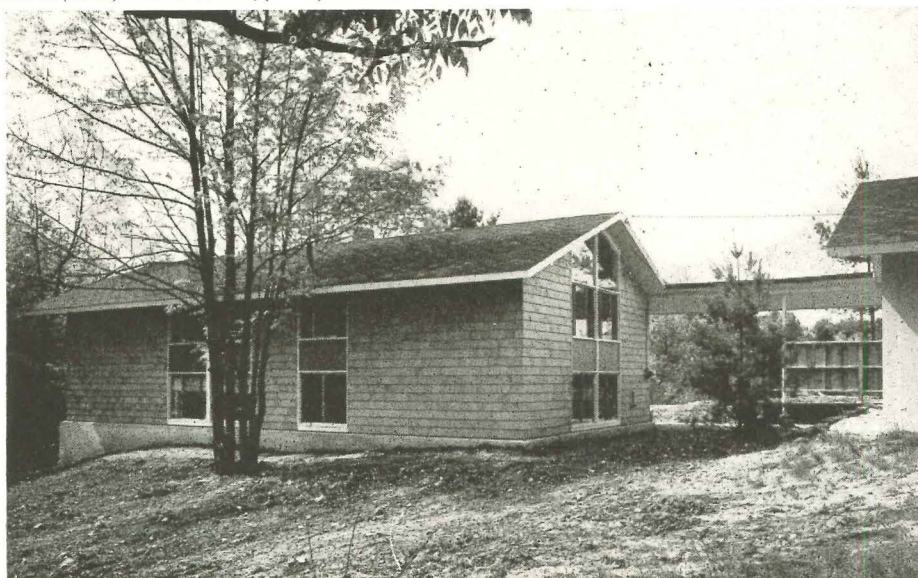
9. Roofing and siding are applied, windows glazed and fitted with plywood panels, walls insulated and interiors finished out. Note roof strip connecting carport, right.
