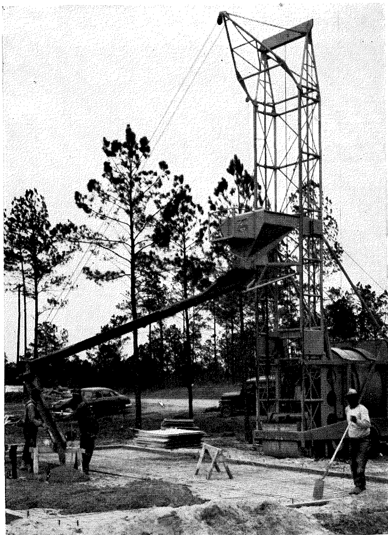
Mobile mixer pours two slabs, is then driven to next pair of foundations
