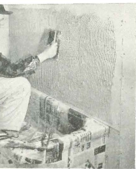
Method of applying thin-set gypsum board is done by who uses a notched trowel.
