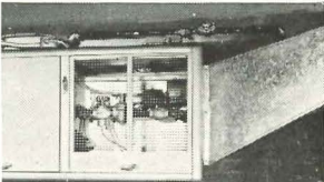
A CENTRALIZED HEATER!!!
