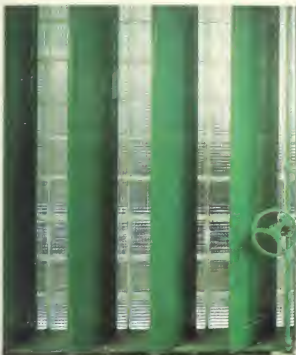
In the conference room, louvers, operated by a wheel, open over glass brick.
