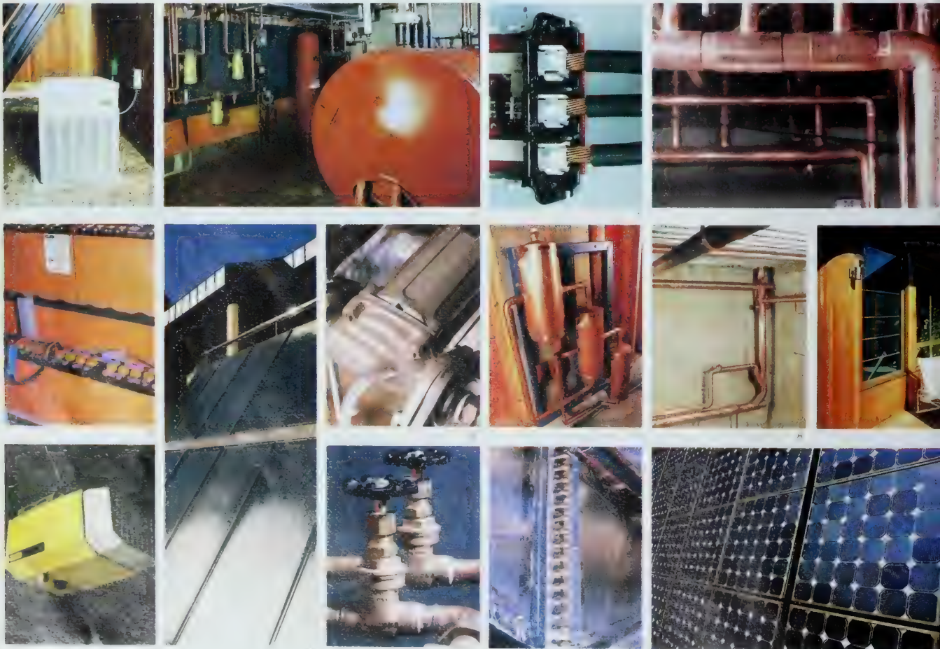
1. Executive Weathertron heat pumps which provide auxiliary heat for the home. 2. Hot water for household use is supplied by the active solar system, Hot-Water-Bank heat recovery unit, and auxiliary electric. 3. Copper liquid solar collectors supply space heating and domestic hot water. 4. Numerous types and sizes of mechanical systems. 5. C&D lead-acid batteries store electricity supplied by Solarex photovoltaic cells. 6. Bronze-bodied pumps keep fluids flowing through advanced mechanical systems. 7. Heat exchangers transfer heat from liquid solar collectors to solar storage tank. 8. Copper Sovent single-stack drainage system takes care of the home's sanitary requirements and provides architectural design flexibility. 9. Polished black copper absorber plate captures sun's warmth and transfers it to freon charged copper heat pipes inserted in copper storage tanks. 10. For convenience and security: Stanley's new Premier garage door opener with safety reverse. 11. Copper liquid solar collectors supply space heating and domestic hot water. 12. Numerous types and sizes of mechanical systems. 13. Filtering air flows over copper fan coil unit through which circulates solar hot water. 14. The Solarex photovoltaic panels satisfy a portion of the home's demand for electricity.
