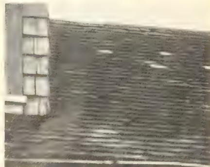
Replace broken, curling, cracked shingles
