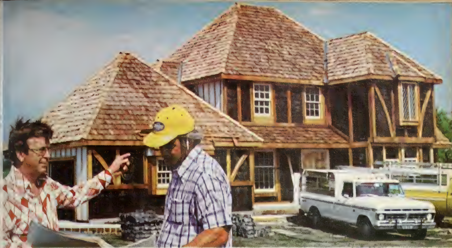
Homebuilder John Huston directs the final phase of construction of another home equipped with Whirlpool products.
