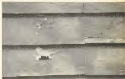
Peeling, blistering paint must be removed
