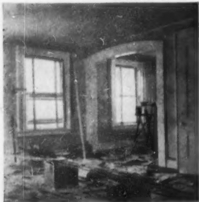
STARTING POINT: off with the old wallpaper in readiness for the new.
