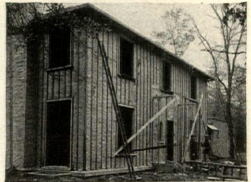
This shows a house insulated with Cabot's Quilt, ready to receive the outside finish. Russell S. Walcott, Architect, Chicago, Ill.
