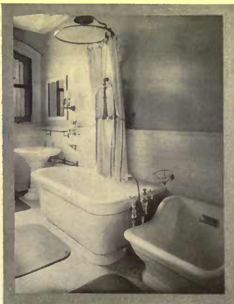
Such unsightly pipe arrangements as those connecting this basin are the result of improper planning
