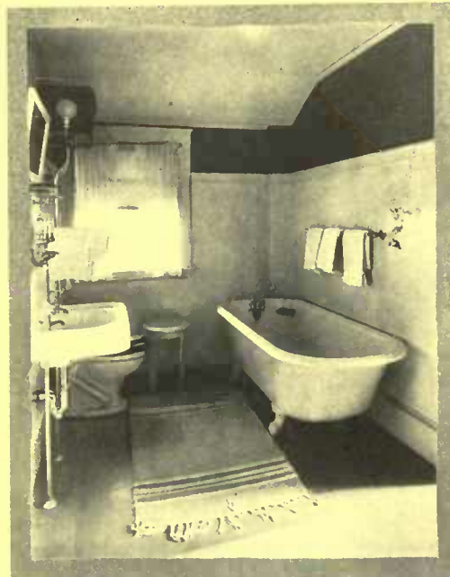
A good type of basin trap. The bend remains full of water which prevents gas from returning into the room
