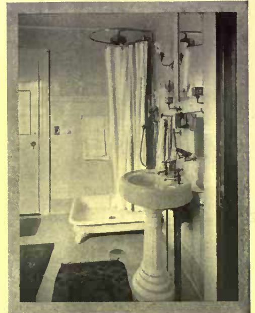
It is difficult to clean the dirt and dust accumulating beneath this shower receptor. It should be flush with the floor
