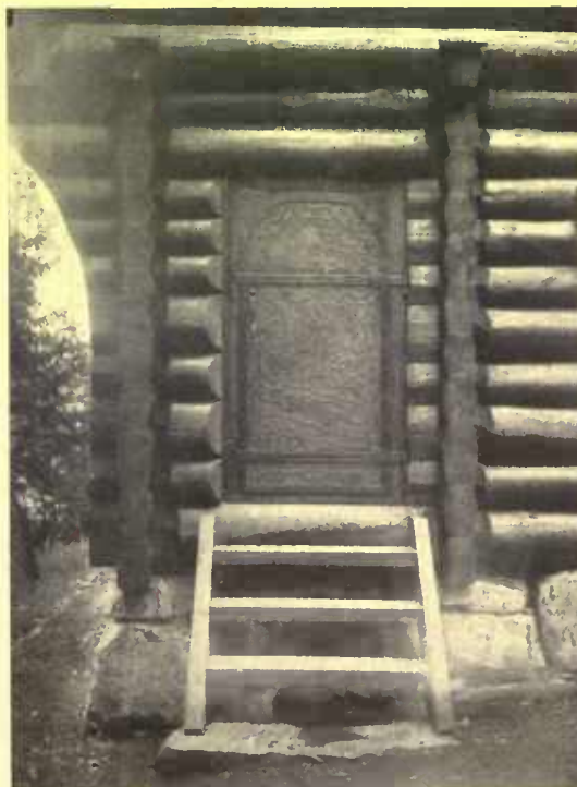
The doorways are decorated with iron work allegorical of the Count's hunting expeditions. Details of these doors are shown above
