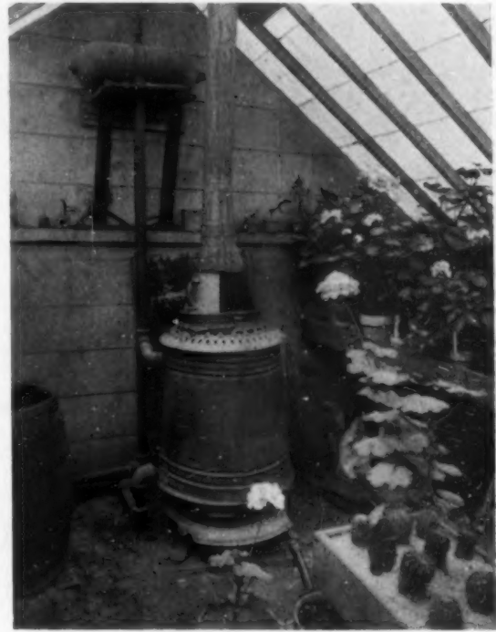
A hot-water boiler from a passenger coach. The system heats 550 sq. ft. of greenhouse with a half-ton of soft coal and cost $25 to instal
