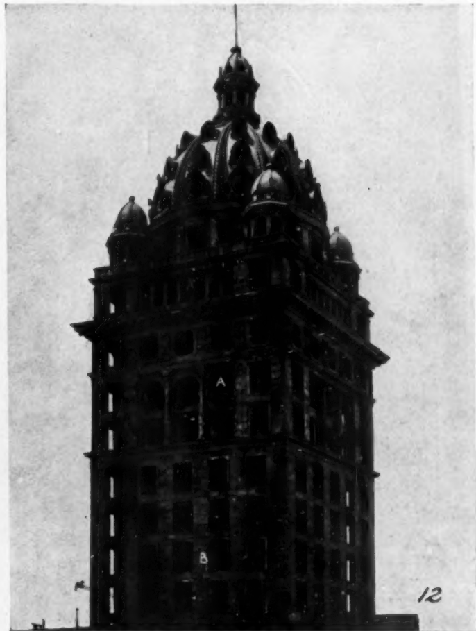
Effect of fire on the Call Building. The terra-cotta dome is intact
