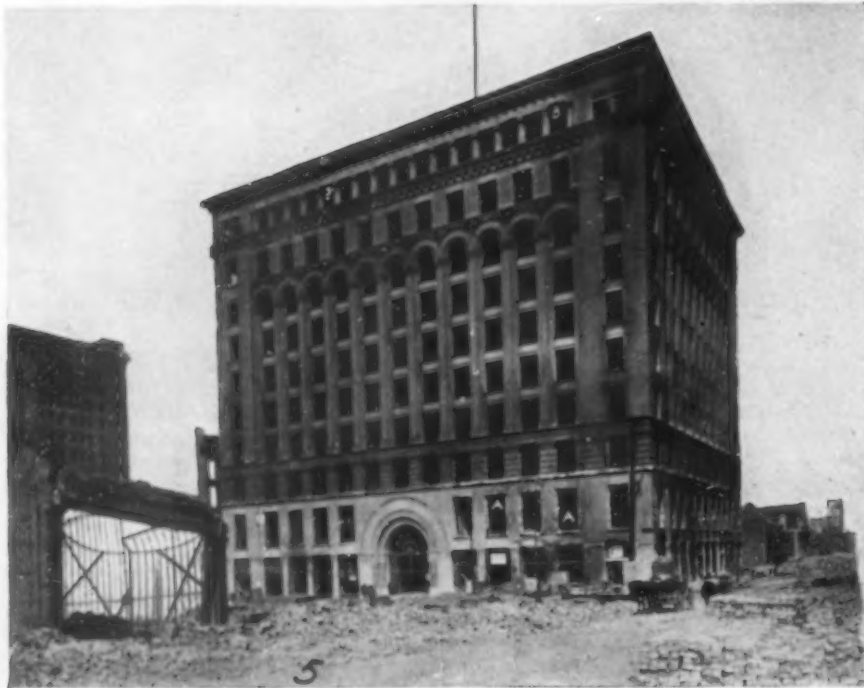
The Mills Building. Stonework scarred at AA, brick above undamaged
