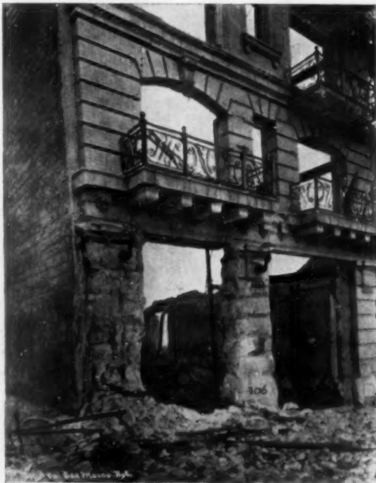
San Marco Apartment. Note the condition of the stone piers while the brick and terra-cotta above are unaffected by fire
