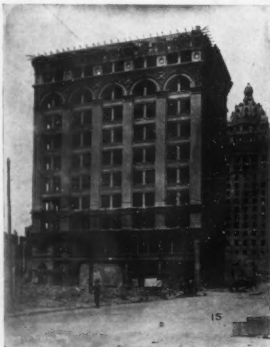
The Aronson Building. Stonework of lower stories damaged and metal cornice gone
