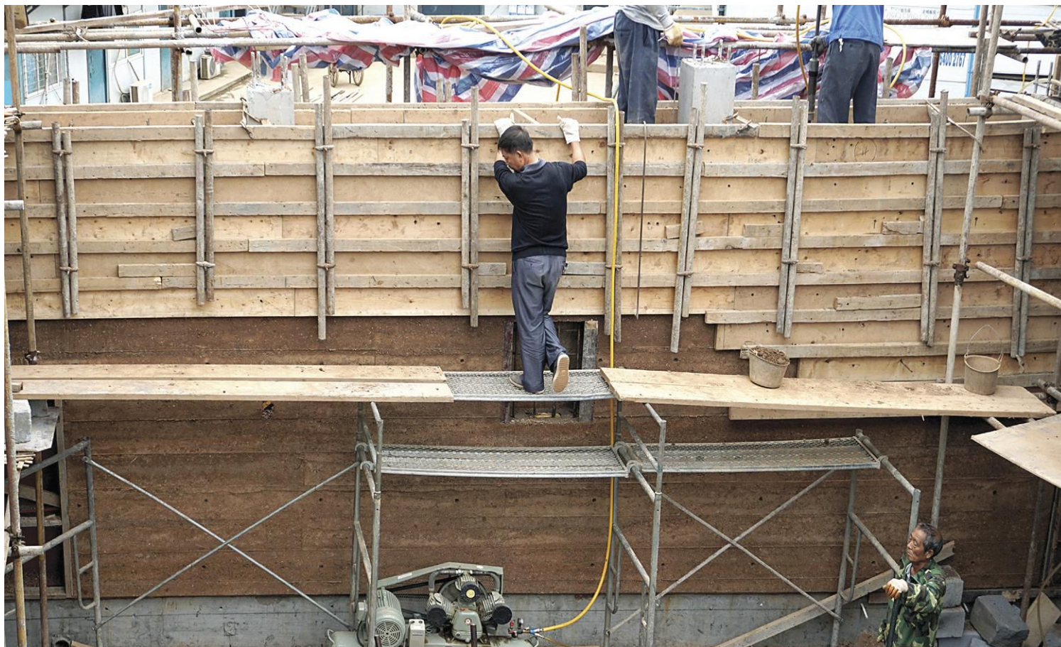
ABOVE BOARD Instead of plywood sheet forms, the museum's walls were poured within horizontally oriented boards to give added texture to the rammed earth's surface.
