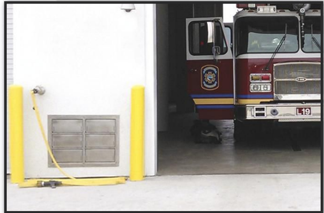
2x3 Multi-frame Smart Vent configuration installed on Fire Station building
