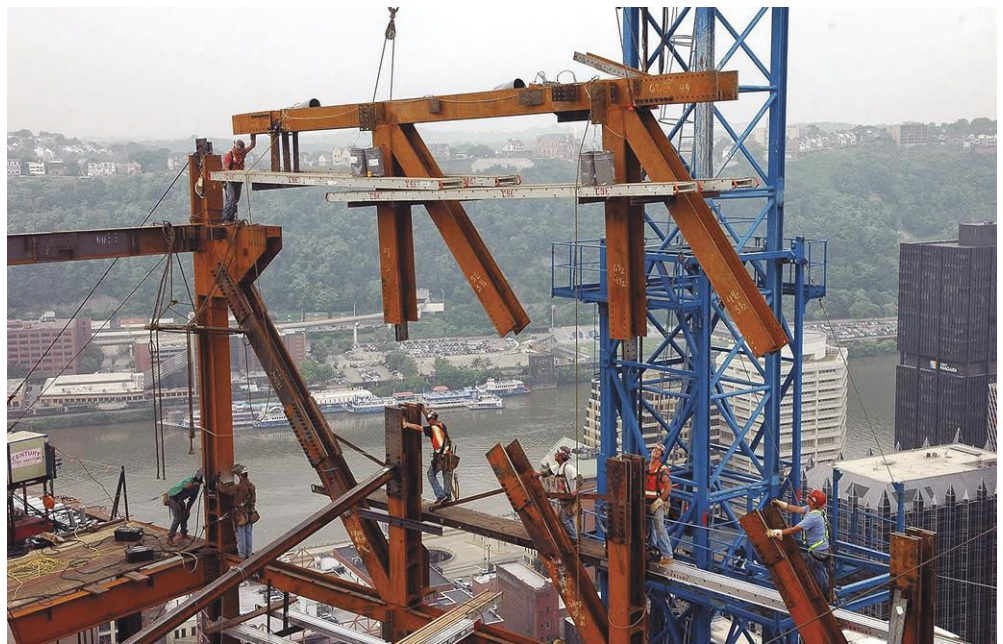
Shown during the erection of the structural steel frame, the new 33-story LEED Platinum Tower at PNC Plaza sits on a five-story podium and houses more than 800,000 square feet of commercial office, auditorium, lobby, cafeteria, parking, and amenity spaces. The superstructure is entirely steel framed using composite steel beams with a steel-braced lateral system. In all, the project uses 8,000 tons of structural steel and 200,000 bolts.
