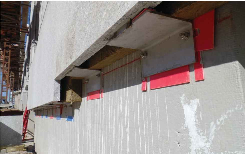
Pictured is a combination gravity and lateral-load anchorage using welded stainless steel anchors.
