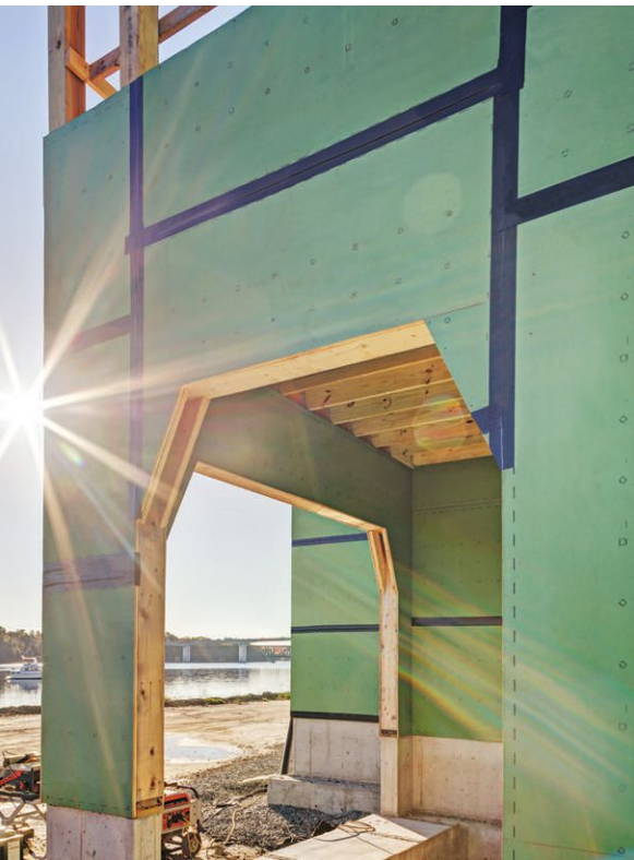
The Whole Building Design Guide and the IBC point out the need to address window openings as an interruption of the air- and water-barrier properties of the exterior sheathing.
