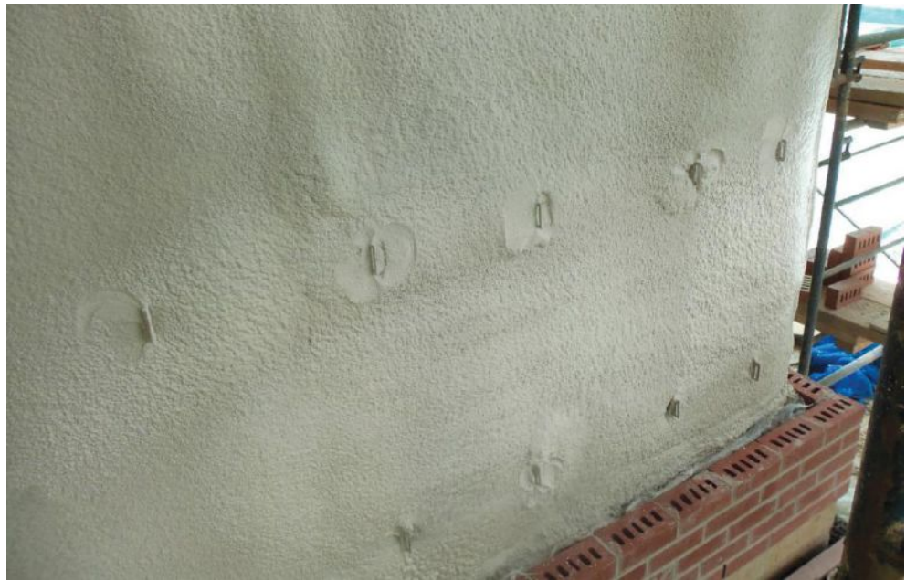
Medium-density, closed-cell spray foam insulation can be applied very precisely in a controlled manner to create a very predictable surface behind cladding.
