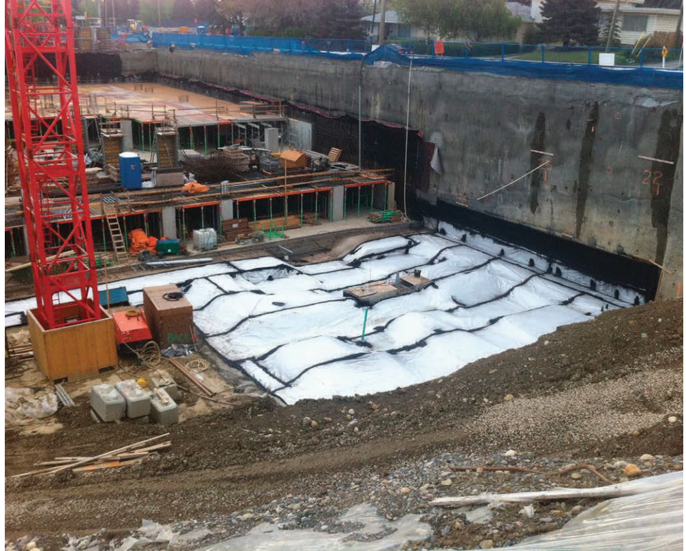
Waterproofing systems can be subjected to stresses beyond hydrostatic pressure alone. The 1-million-square-foot West LRT Tunnel constructed in Calgary, Alberta, Canada, during the winter time is an example of the need for waterproofing to resist stresses from cold temperatures and possible seismic activity.
