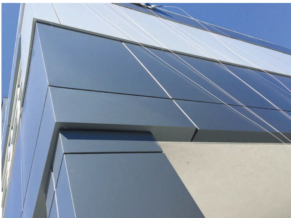
Exterior ACM cladding examples include the Brooklyn Bridge Pierhouse (left) in Brooklyn, New York, and 92-77 Queens Boulevard (right) in Queens, New York.
