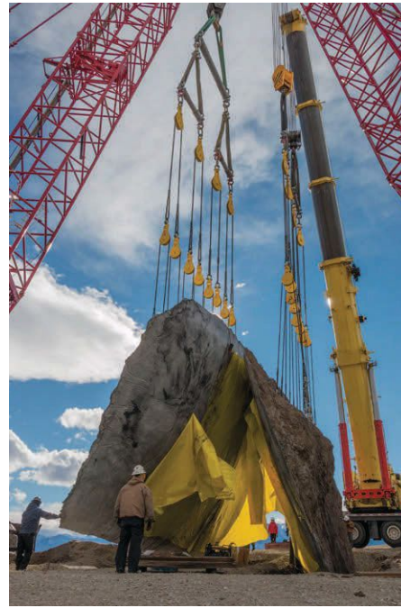
INVERTED PORTAL BY ENSEMBLE STUDIO UNDER CONSTRUCTION AT TIPPET RISE ART CENTER IN MONTANA.
