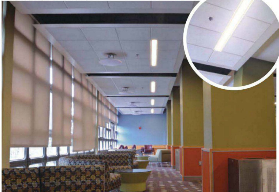
Linear LED luminaires provide soft lighting for Boston University Rich Hall residence in Boston, Massachusetts.
