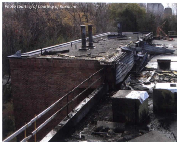
Roofing insulation stands up to an intense four-alarm fire at York University in Toronto, Canada. Noncombustible stone wool insulation prevented the fire from spreading, avoiding damage to property and possibly any human loss.
