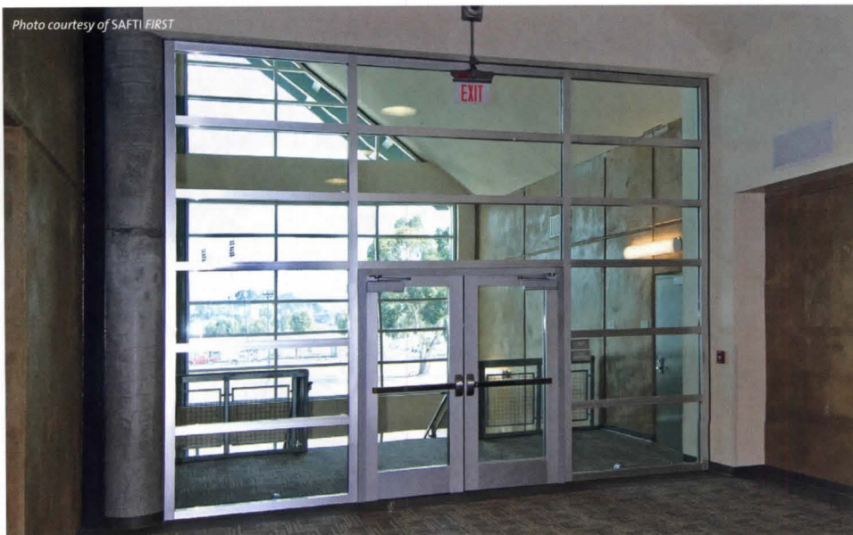
Fire-resistive glass assemblies can create a sense of openness, add natural lighting, and increase the visibility to safe pathways.
