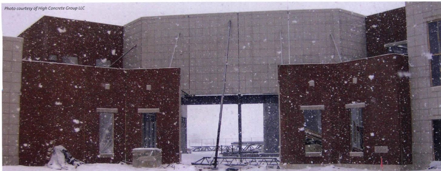
Precast concrete can be quickly erected even in the winter, as shown in construction photo of Willow Creek Elementary School in Fleetwood, Pennsylvania. Designed by AEM Architects Inc.
