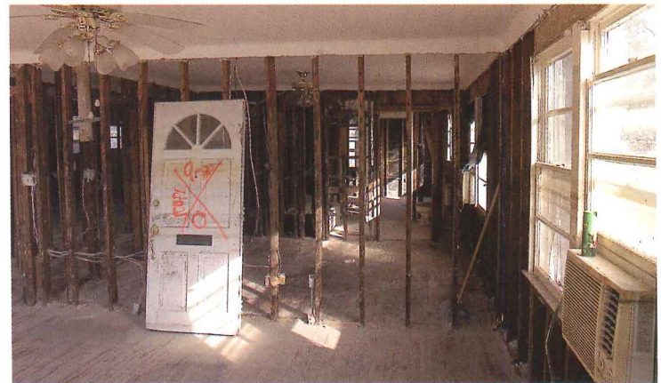
Views near the 19th Street Canal, in the city's northwest, resemble a bomb's aftermath (top). Elsewhere, a home is being gutted and repaired (bottom).
