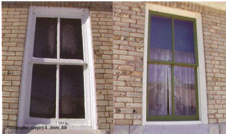
Window before and after restoration by SmithGroup at Old Mackinac Point Light Station
