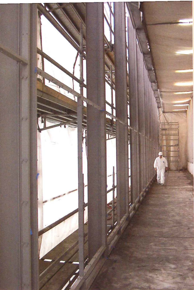
New frames and tops are in place, awaiting installation of the glass (above). The difference between the original detail (top right) and the new one (right) is very subtle.
