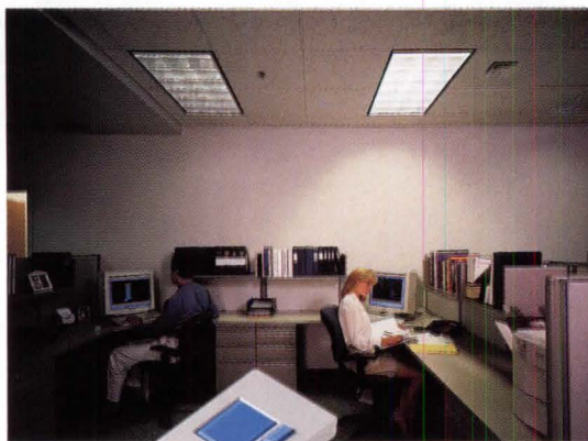
Systems that permit individual control of lights exist (here, a system by Lutron), but Berkeley's study uses new sensors that will make them cheaper.
