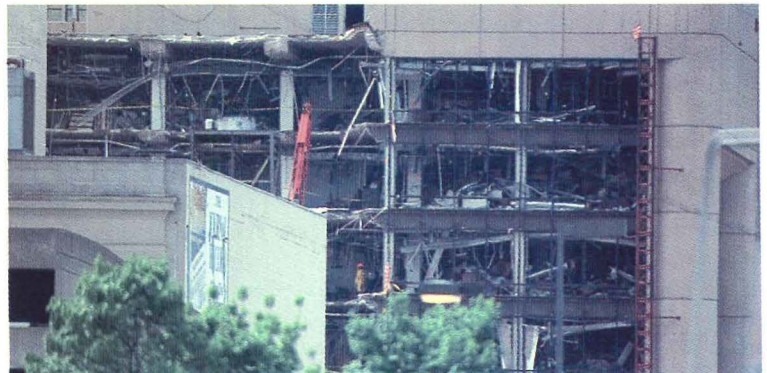
Structural damage and broken glass were major contributors to death and injury for both the targeted buildings and the surrounding area in the 1995 bombing of the Murrah Federal Building in Oklahoma City.
