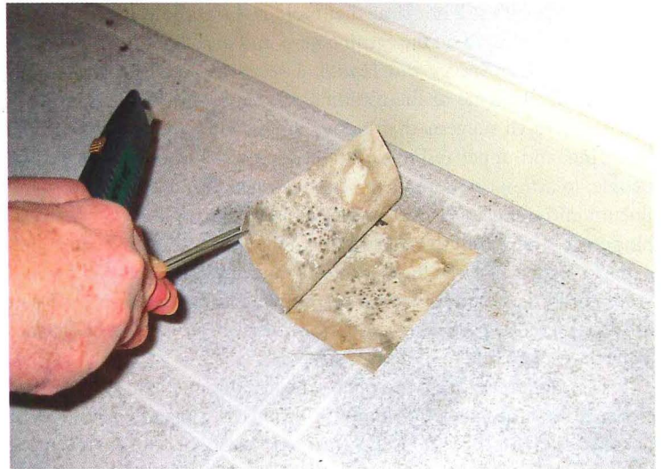
Mold grows under sheet vinyl covering a concrete floor in the Midwest because a vapor barrier had not been placed below the slab during construction, thus allowing ground moisture to penetrate the concrete.
