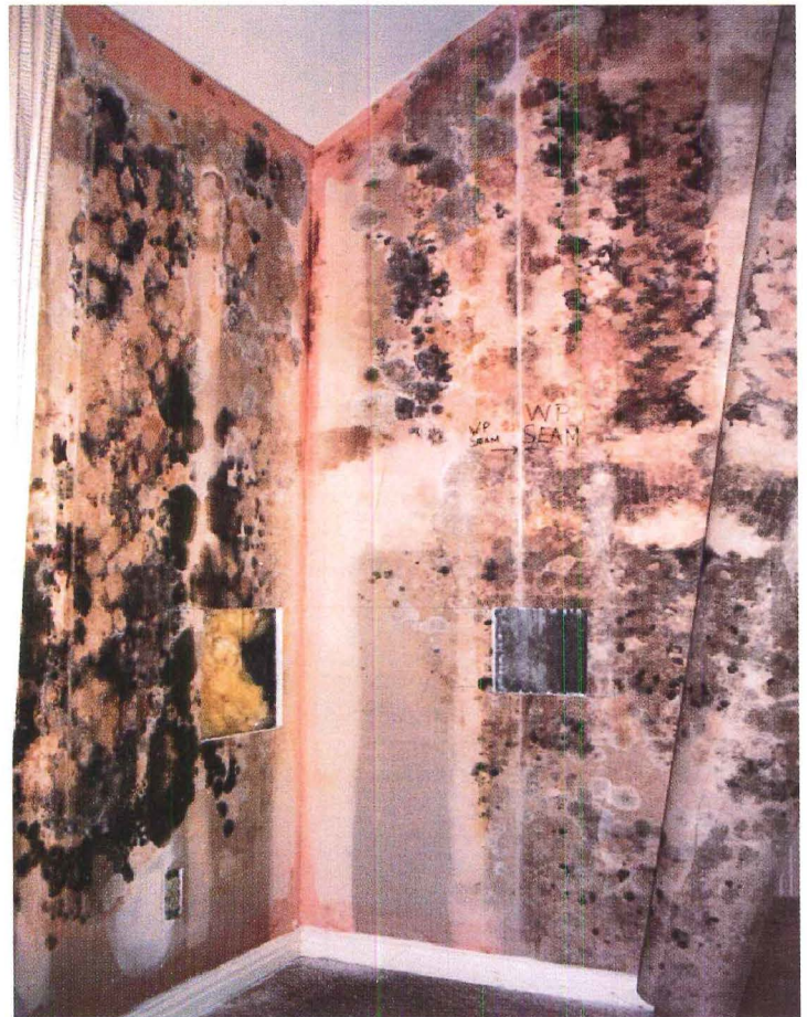
Mold flourishes on wallboard behind impermeable vinyl wall covering in a Florida hotel. Condensation forms when moist warm air from outdoors meets cooler spaces indoors. The vinyl traps the water, which is key to mold growth.
