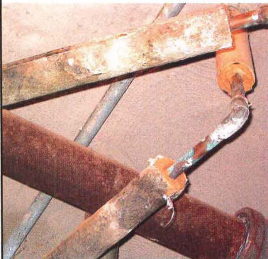
Moisture control is the key step in halting mold growth in buildings (171).
