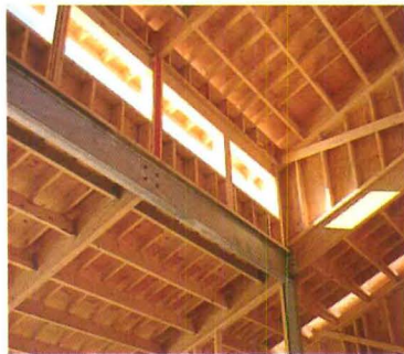
Clerestory windows help provide balanced day lighting. Environmental Experiment Center (EEC) at the Science Museum of Minnesota in St. Paul.
