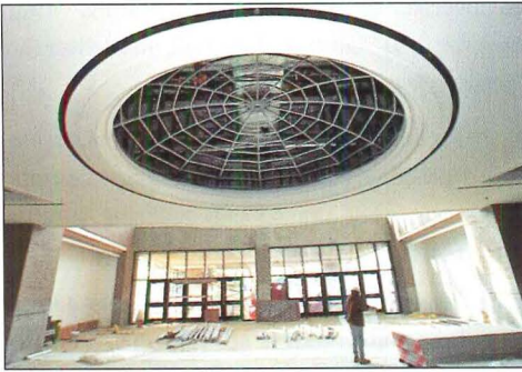
The USG Drywall Suspension System saved hundreds of man-hours and ensured perfect results on the construction of 19 domes in Regent Auditorium, Pensacola.
