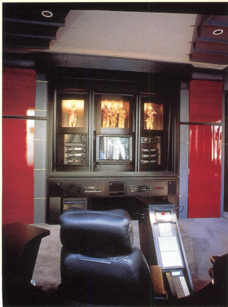
Command Center: A keypad "super station" in a project designed by Holt Hinshaw Architects controls lighting, mechanical systems, even the swimming pool as well as a sophisticated home theater system. The red-stained Okume-wood veneered panels conceal mechanically ventilated space for 17 amplifiers.
