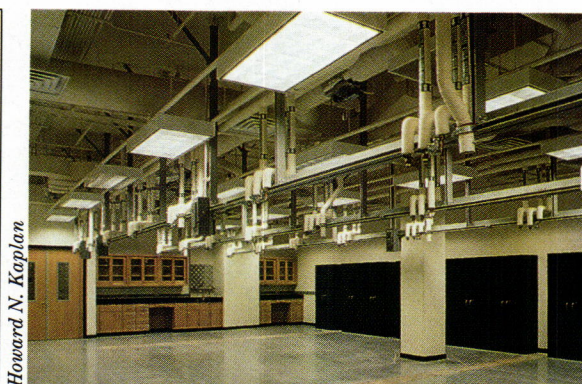
4. At Engineering Unit II at University of California, San Diego, exhaust fans are placed in locations remote from air intakes. Ove Arup & Partners California, engineers; Zimmer Gunsul Frasca Partnership, architects. 5. Materials and Life Sciences Building at Northwestern University (by Perkins & Will) has large rooms with overhead piping for equipment flexibility.
