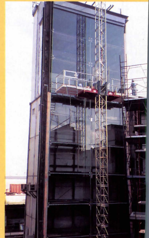
Testing of a 21-by-64 foot all-glass curtain-wall mockup at the Construction Research Laboratory.
