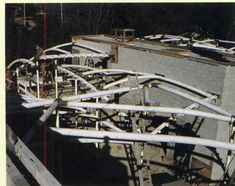
The south terrace (top drawing) and view north from the entrance (bottom drawing) are shown above. Steel elements, which Holl calls “noddles in space,” form a frame of doubly curved metal roofs, shown under construction (above).
