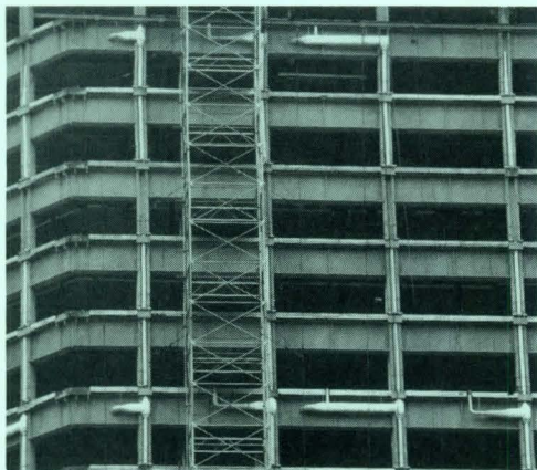
Ducts from the core for the perimeter induction system penetrate spandrel beams every fifth floor, feeding up three floors and down two. The mechanical engineer, Joseph R. Loring & Associates, detailed the ductwork for tight space (see detail below).
