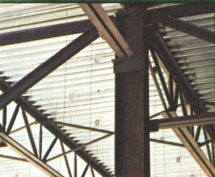
The efficiency of Vulcraft's standardized column joists speeds up steel erections and saves costs.
