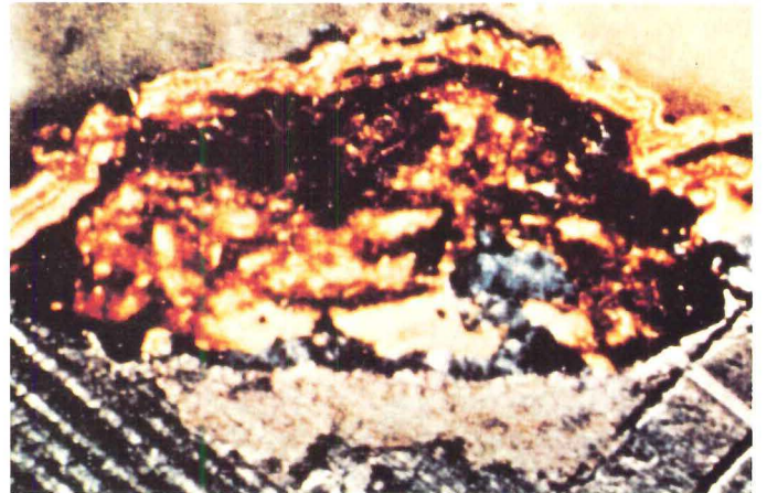
This magnification shows how rust expands as steel corrodes.
