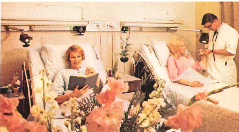
One example of Keene hospital lighting is this console containing fluorescent fixtures, plus examination and reading lamps.
