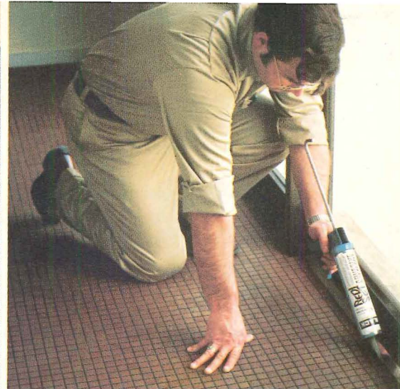
seal around tilework,
