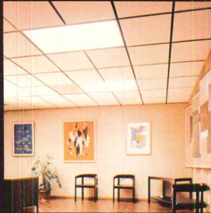
Pyrotec recessed edge acoustical panels in office waiting room
