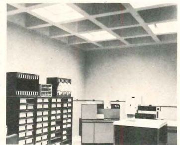
LIGHTING SYSTEM / H.I.D. 400-watt mercury luminaires recessed on 6-ft centers in alternate coffers comprise the system. In the installation shown here, nine fixtures achieve a lighting level of 240 footcandles. ■ Holophane Co., Inc., New York City. Circle 305 on inquiry card
