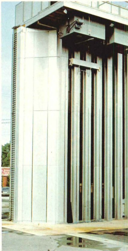
(Left)—Testing a prototype of the wall system by Cupples Products Division, H. H. Robertson Co., checked out the wind loading and thermal performances.
