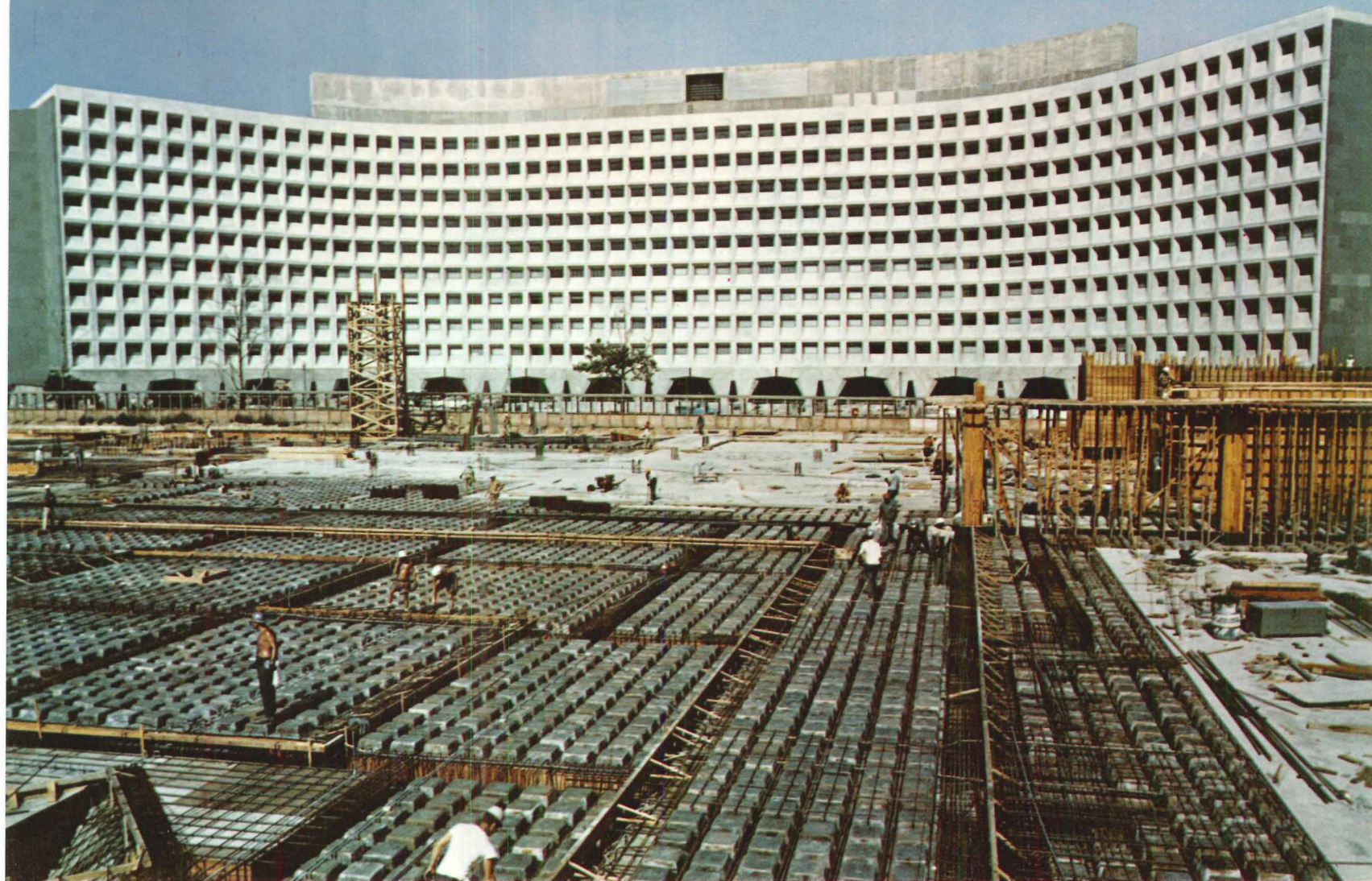
Foreground: Construction of Nassif Office Building, Washington, D.C. 2,000,000 sq ft of Ceco Steeldome Services David Nassif Associates, owner / Edward Durell Stone, architect Universal Engineering Corp., engineers John A. Volpe Construction Co., Inc., contractors Kirk Lindsey, Inc., concrete contractors (Background—National headquarters building of HUD also utilized Ceco's experience in forming reinforced concrete joist construction for central core.)
