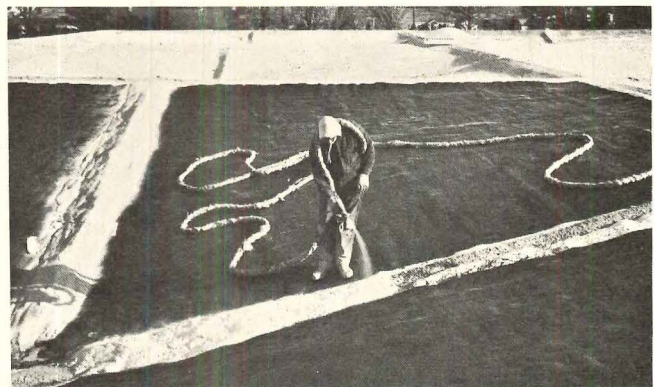
Good resistance of rigid urethane to thermal stress was critical factor in sealing expansion joints between parabolic shell sections on roof.
